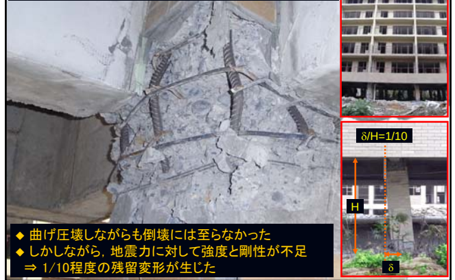
(3) 柱頭・柱脚破壊／Hinges at Column Ends
