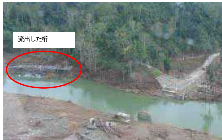
写真-5 ロッカチャ橋梁 (No. 9) の桁の流出 (Photo by UN) (5° 22' N, 95° 16' E)
