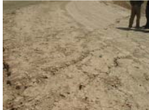
Figure 5.14. Cracks crossing the body of dam at its left abutment
