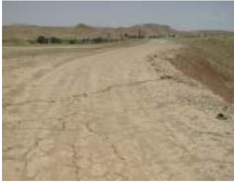
Figure 5.13. Cracks crossing the body of dam near its right abutment
