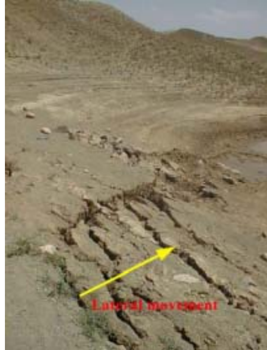
Figure 5.17. Lateral movement of left bank at upstream side
