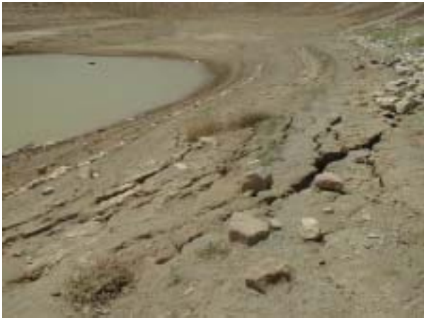
Figure 5.12. Instabilities at upstream slope from a closer view
