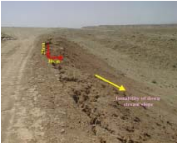
Figure 5.10. Instabilities at upstream slope
