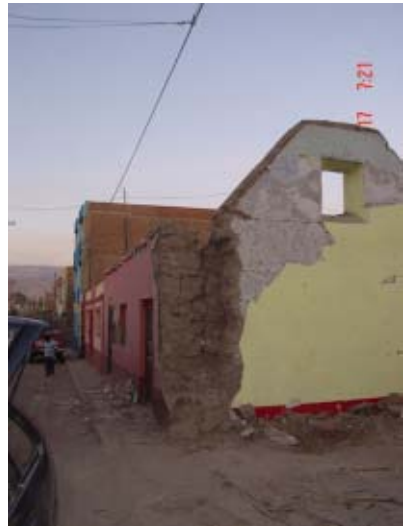
Photo 5.14 Weak adobe house corner
