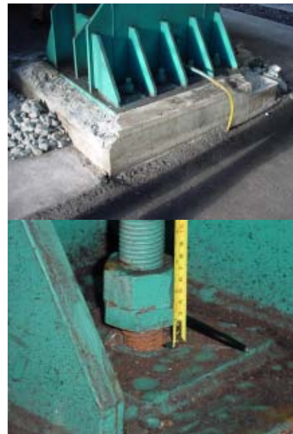
Photo 5.2.5 Yielding of anchor bolts in 8-bolt layout column base
