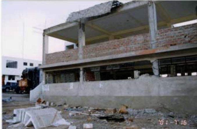
Photo 5.7. In the first floor, deep beams are provided in one direction only whereas in the second floor they are provided in both directions.
