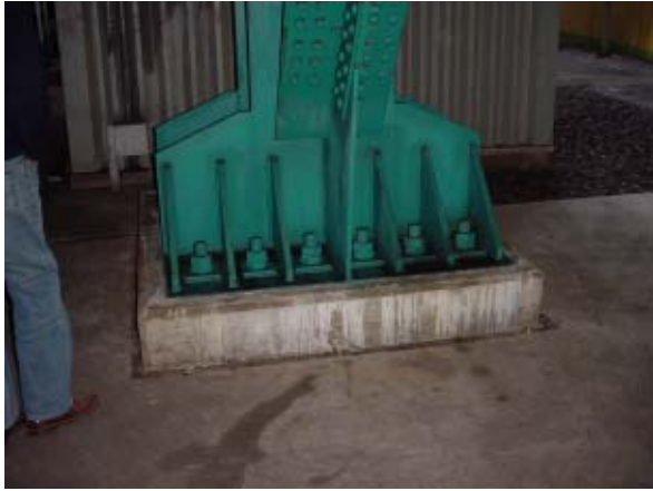
Photo 5.2.6 Almost no damage is seen at interior column anchorage, 12-bolt layout
