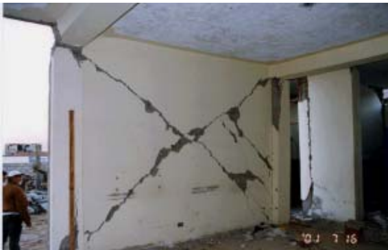
Photo 5.11. In-plane failure of a masonry infill.
