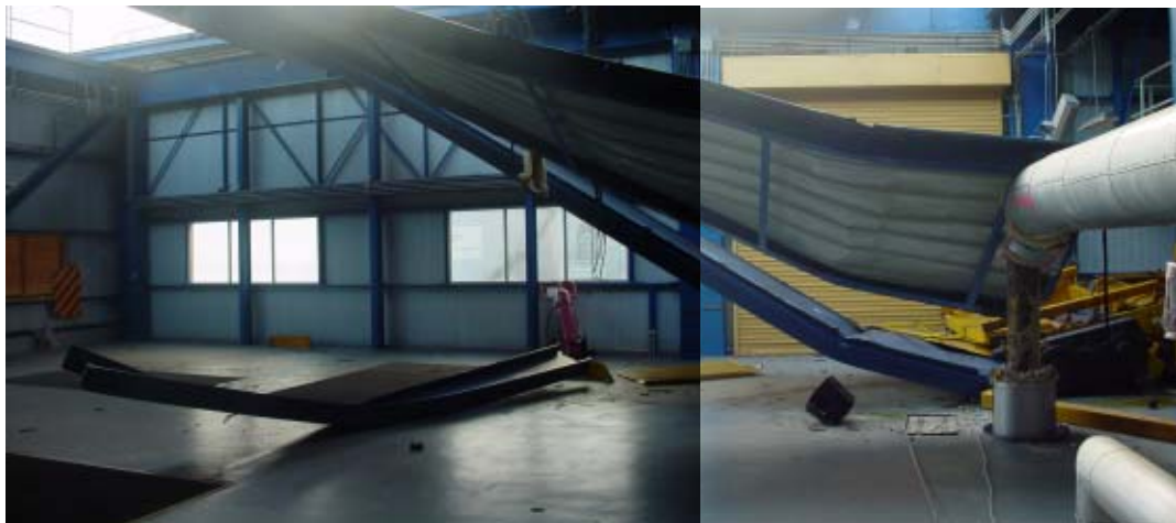
Photo 5.2.12 Steel sub-beam supporting roof panels was completely broken
