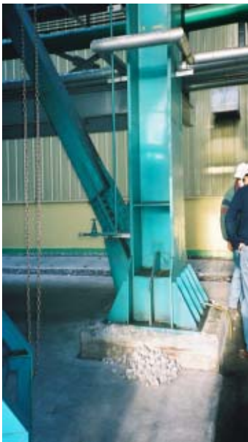
Photo 5.2.4 Damaged column anchorage
