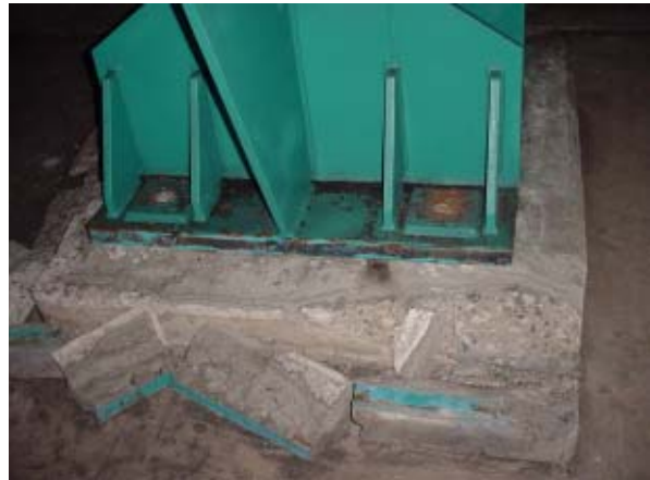
Photo 5.2.7 Completely broken anchor bolts in 4-bolt layout column anchorage
