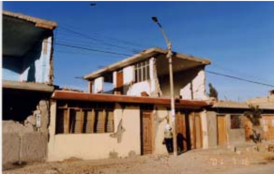
Photo 5.11. Out-of-plane failure in an unreinforced masonry dwelling
