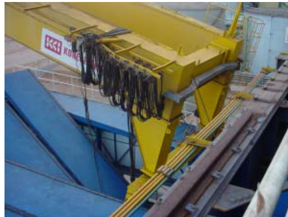
Photo 5.2.11 Fasteners that fixed crane rail were completely broken
