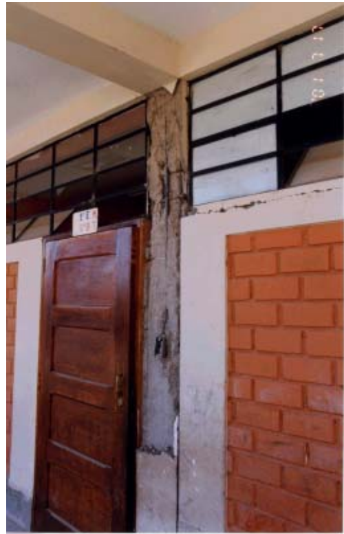
Photo 5.9. Detail of concrete cover spalling due to insufficient cover and utility pipe in the column border.
