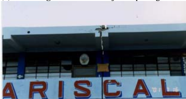
Photo 5.10. Pounding between two buildings at Andres Avelino Caceres School, Tacna.
