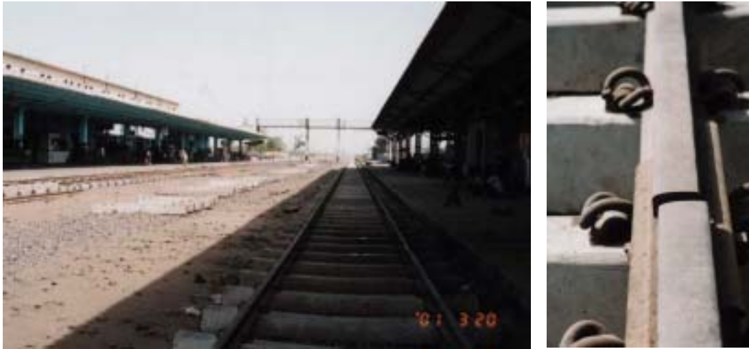
Figure 5.3 Railway lines in Gandhidham station and a close-up view of distorted rails
