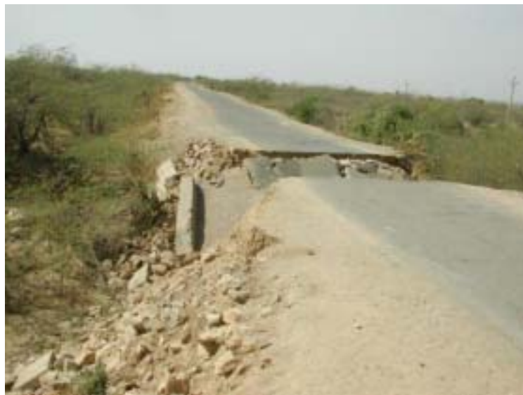
Figure 5.10 Collapse of a minor roadway bridge (Oyo corporation)
