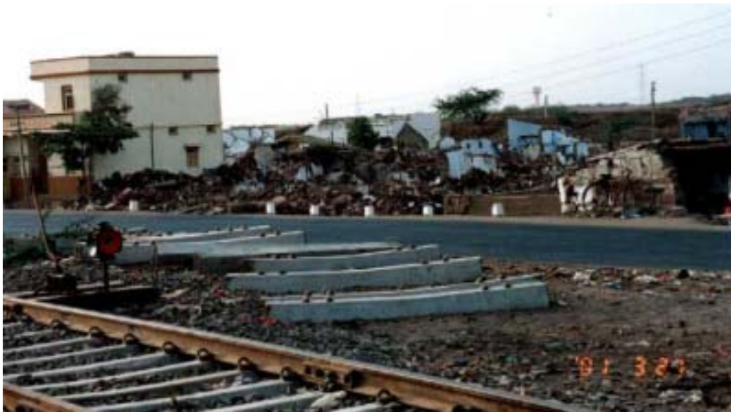
Figure 5.2 Restored railway line in Ratnal (note the damaged railway ties)
