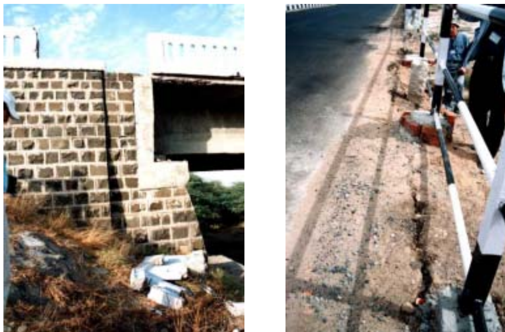
Figure 5.11 Damage to parapets and settlement of bridge over Macchu River
