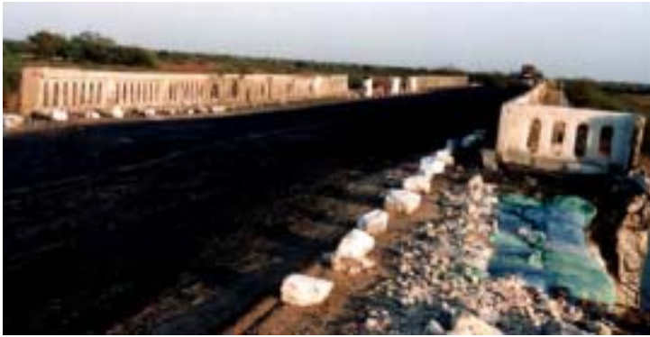
(a) Damaged bridge on Kankawati River
