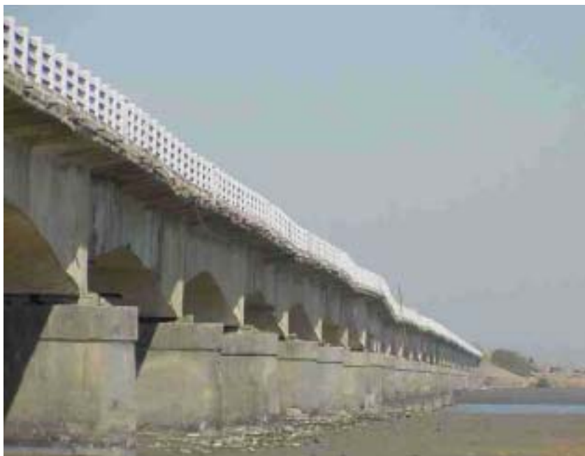
Figure 5.12 Damage to Hadakiya Bridge (Suraj Bari)
