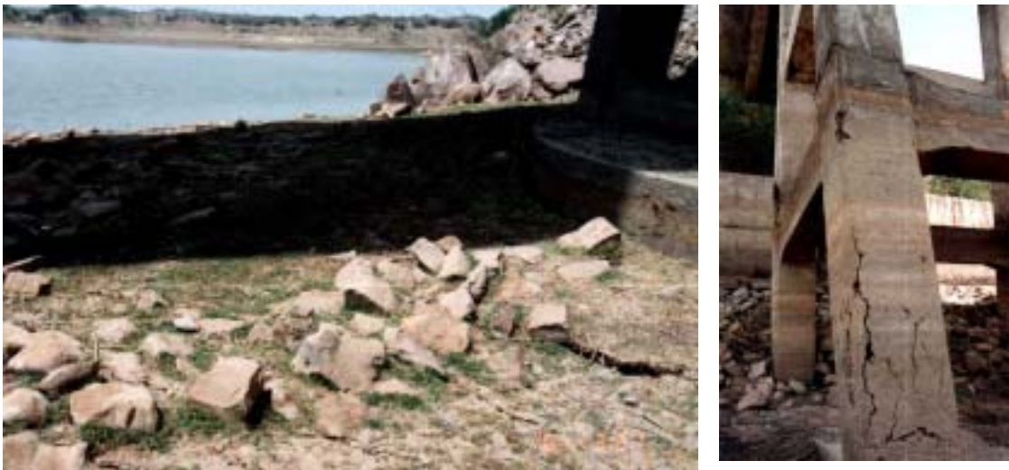
Figure 5.14 Settlement of ground around a pier of Rudramata bridge and its damaged state (note also the fallen rock blocks in the vicinity of the pier)
