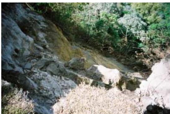
Figure 2.57. Slope failure at Site VI
