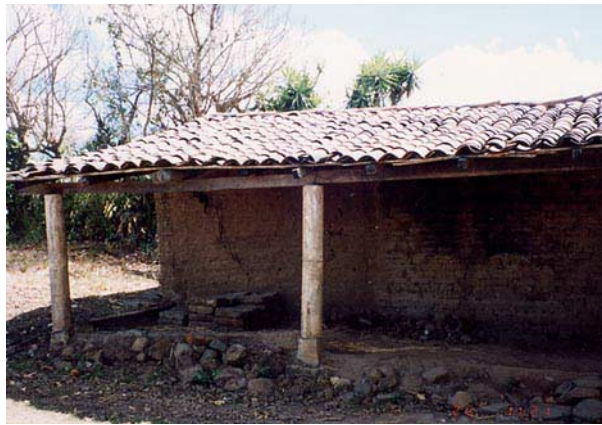
Figure 2.66. Bahareque house near San Vicente landslide
