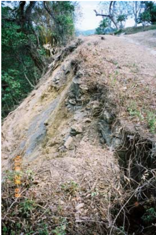
Figure 2.54. Slope failure at Site III
