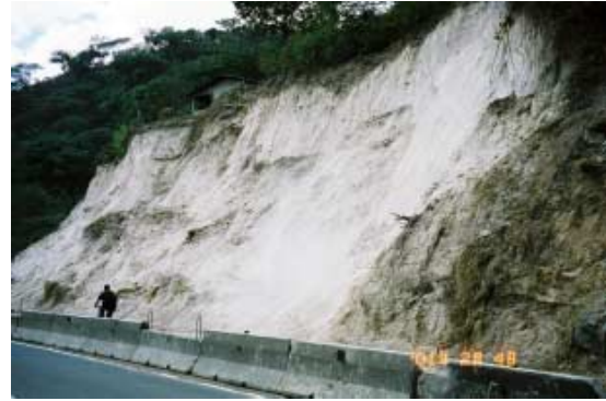
Figure 2.60. Exposed failure surface of pyroclastic flow sediment.
