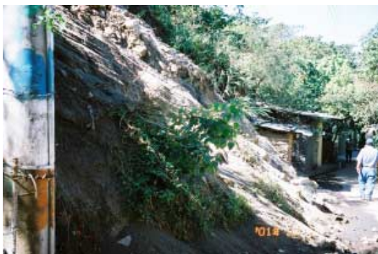
Figure 2.62. Slope failure on weathered tuff
