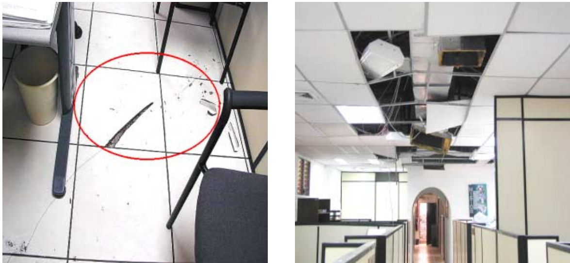
Figure 4.12 Damage to the headquarter building of “El Salvador Electricity Transmission Company” (ETESAL)
