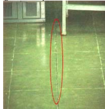
Figure 4.11. Tension crack along a joint between tiles (Switchyard, Sonsonate Substation)
