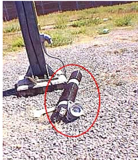
Figure 4.3. Broken bushing for a lightning rod (Nejapa Substation)
