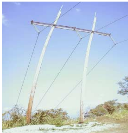
Figure 4.15. Tilted plane frame of the Nuevo Cuscatlan–Santo Tomas 115 kV line
