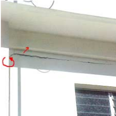
Figure 4.10. Lateral crack beneath a beam (Switchyard, Santo Tomas Substation)
