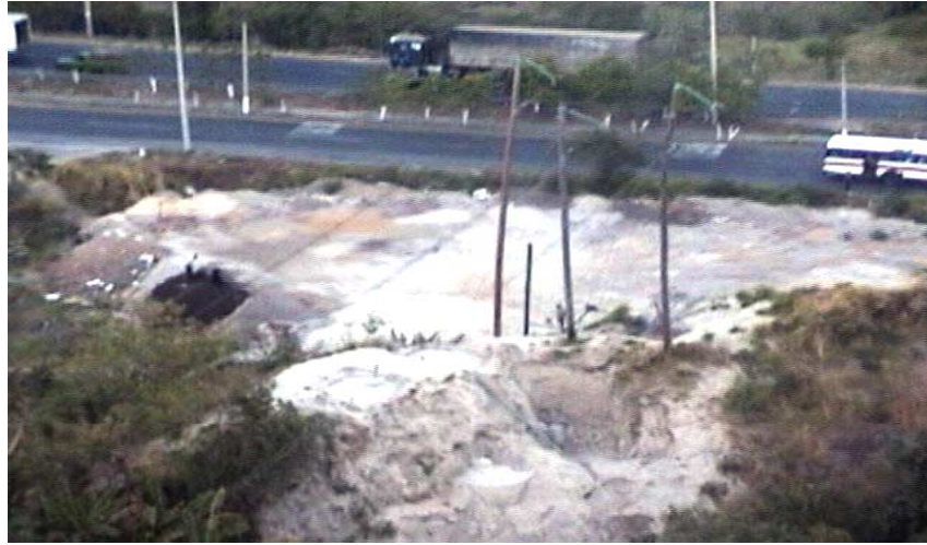
Figure 4.13 Damage to wooden poles for transmission cables. (San Martin– Nuevo Cuscatlan Transmission Line)
