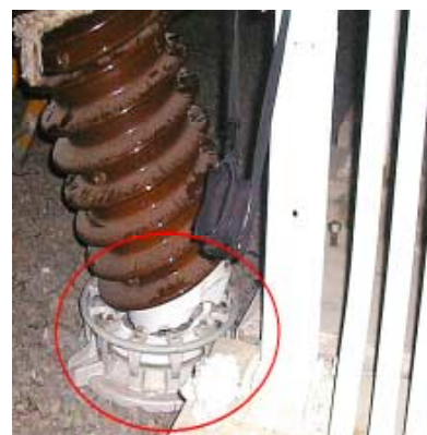
Figure 4.5. Broken support of interrupter (Nejapa Substation)
