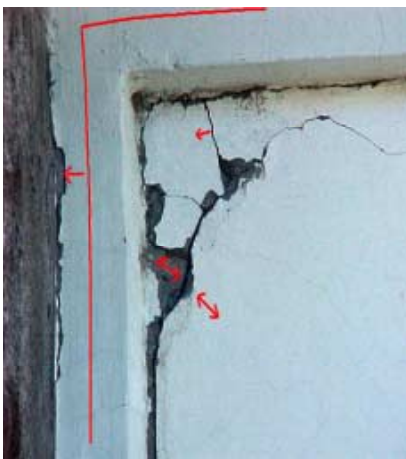
Figure 4.8. Cracked corner of a wall
