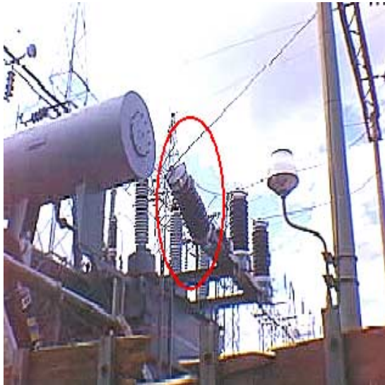
Figure 4.2. Broken bushing for a transformer (Soyapango Substation)
