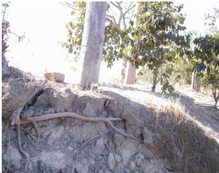
Figure 4.17 Roots cracking soils (Nuevo Cuscatlan-Santo Tomas Line)
