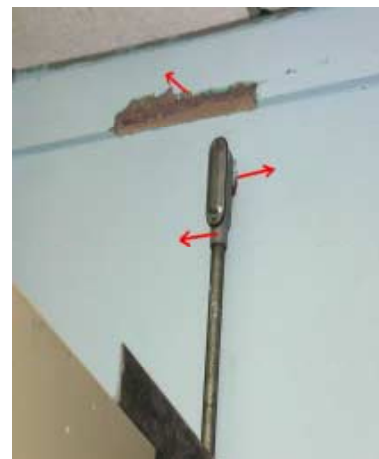
Figure 4.9. Spalled concrete beam
