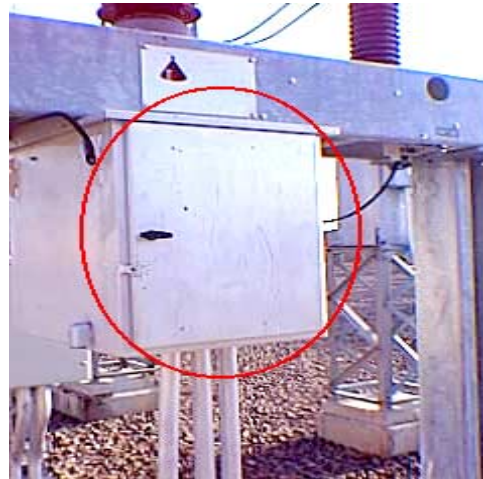
Figure 4.7. Main switch board
