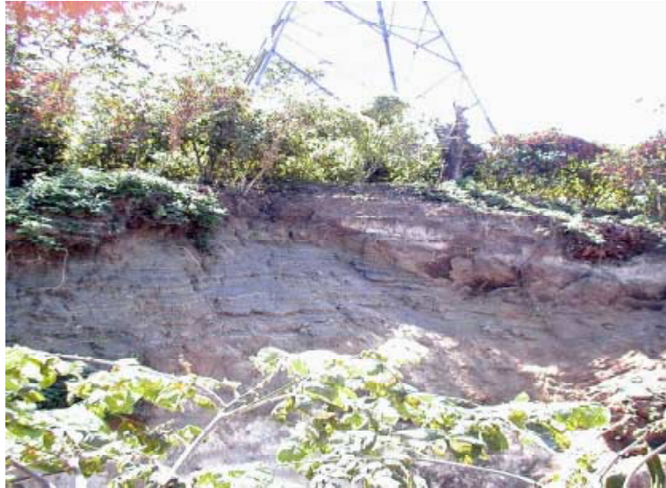
Figure 4.16. A slope failure about 4m off a transmission tower: Foundations of the tower narrowly escaped from being carried off. The failure surface extended over 8 meters height and 12 meters wide (Nuevo Cuscatlan-Santo Tomas Line)
