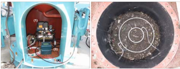
Gas injection system
