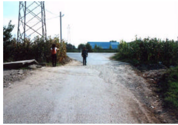
Figure 4.11 Faulting in Kullar village
