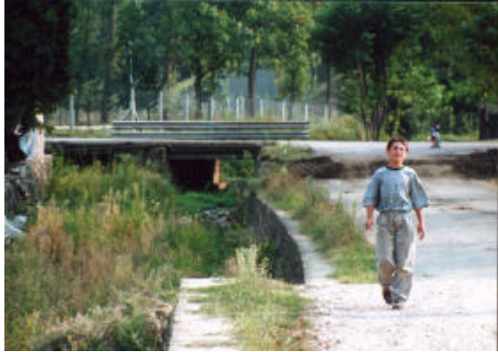
Figure 4.12 Faulting in Arifiye
