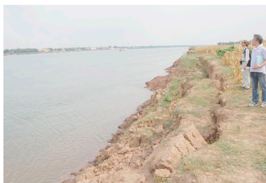
Photo 9: The State of Erosion at the Right Bank of the Mekong River
