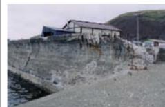
Prior to corrective measures, these revetments were in a dilapidated state with deteriorating concrete.
