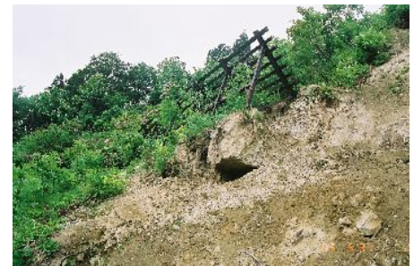
Damaged snow barrier
