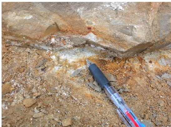
Tuffaceous sandstone of slipped surface
