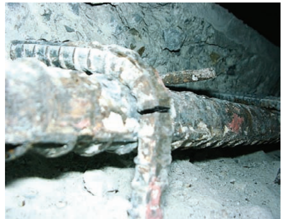
Photo 2.2 - Failed Steel Bar
