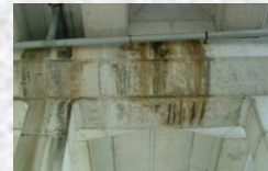
Corrosion of rebar at water splash point (RRR,68(4),22-25,2011)
