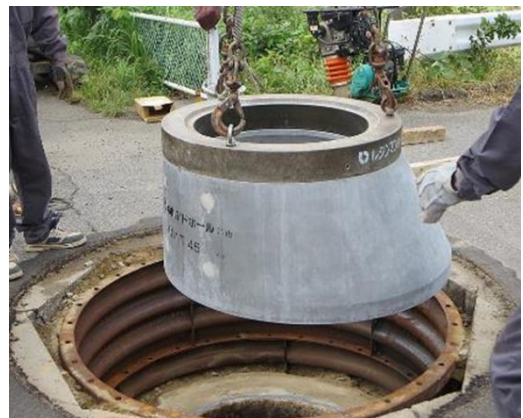
<Acid resistance> Slanted manhole
