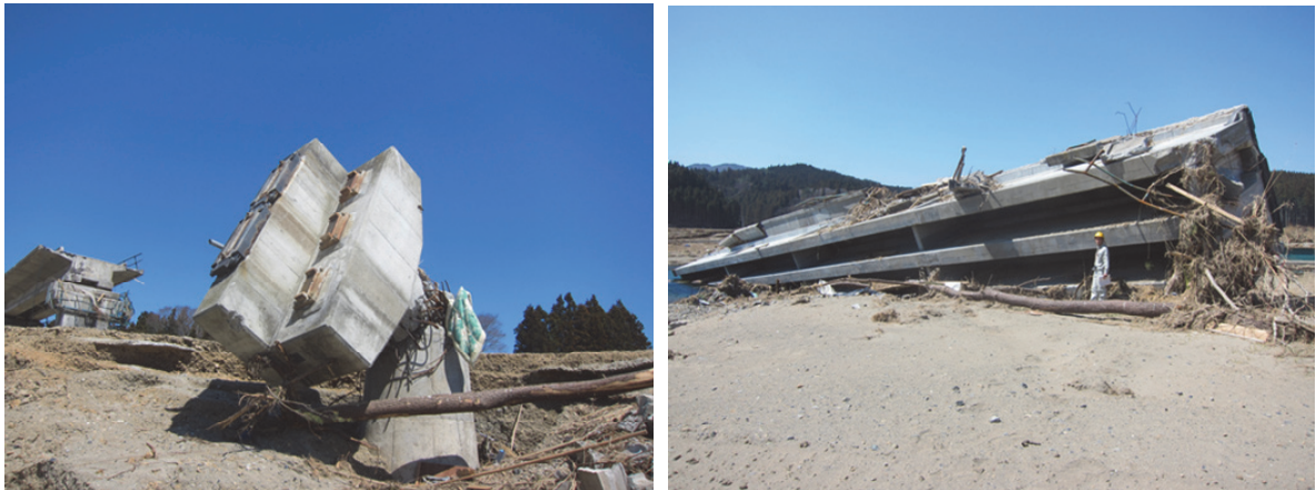
Figure 10 Overturned PC girder and damaged piers of railway bridge
