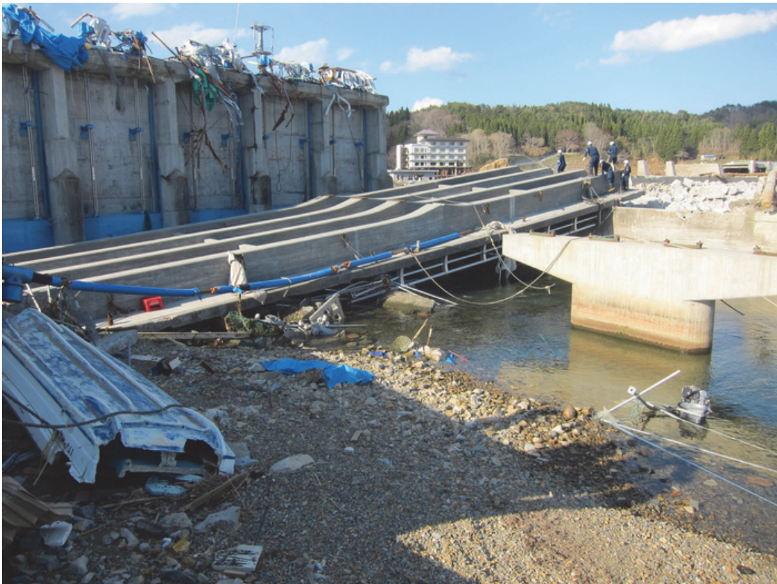
Figure 11 Overturned girder in the case of a low bridge near a sluice gate (Minato-hashi)
