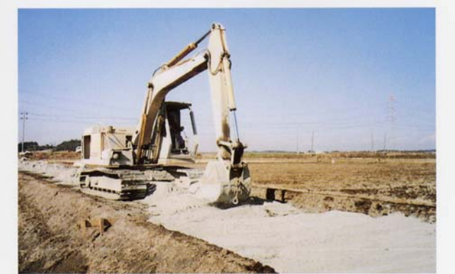
Soil stabilization using Geoset Eco, cooperatively developed by the Ministry of agriculture, Forestry and Fishery of Japan and Taiheiyo.
