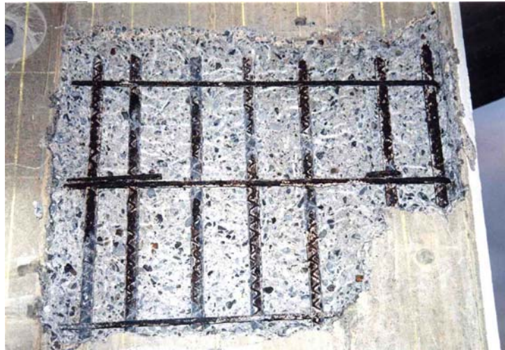
Photo2 Verification of corrosion of rebar by removing cover concrete
