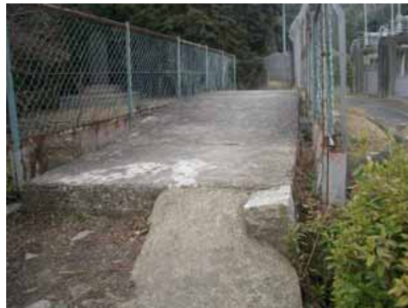
Surface of Hinooka RC11 Bridge (The surface is still in excellent condition.)
