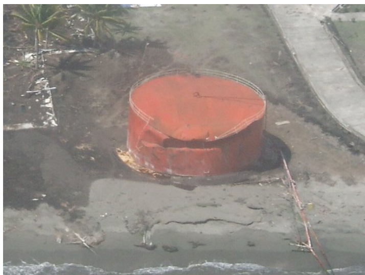
Photo 9.3 Buckled and settled tank at Meulaboh
