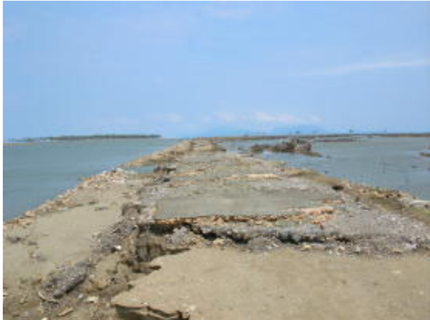
Photo 11.18 Washout of Pavement and Soils
