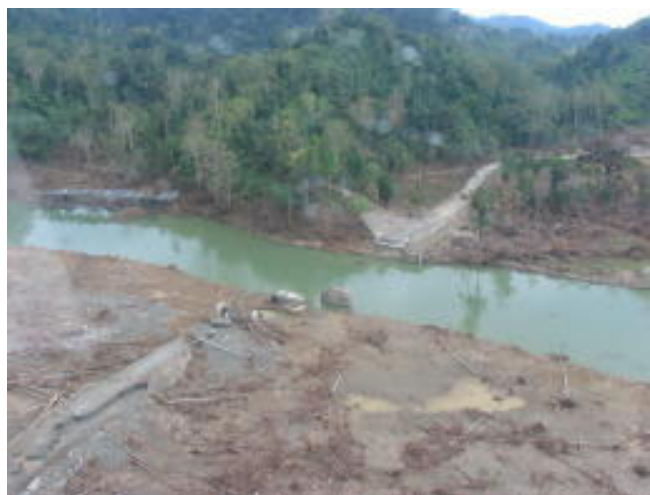
Figure 11.28 Washout of Truss Bridge (5) (courtesy of Aceh Provincial Government)
