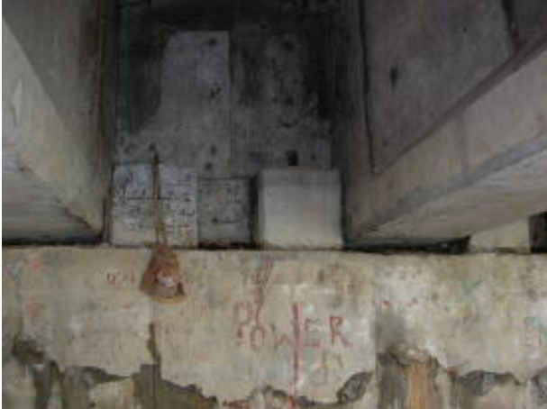
Photo 11.14 Slight Damage to Shear Keys
