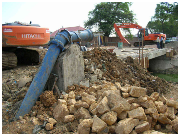
Photo 11.2 Collapse of Water Pipes
