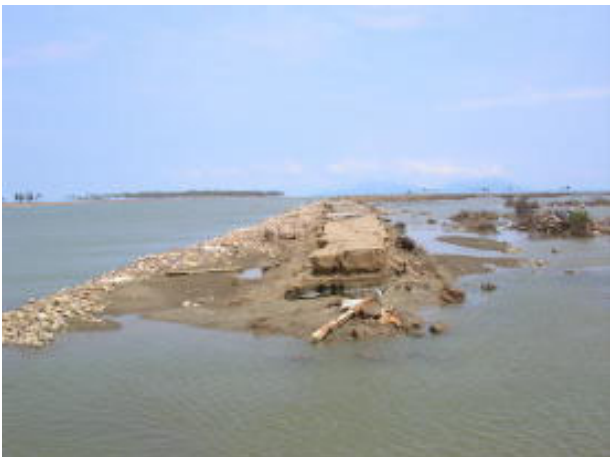
Photo 11.17 Washout of River Dike
