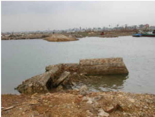
Photo 11.3 Complete Washout of Bridge (being reported as wooden bridge)
