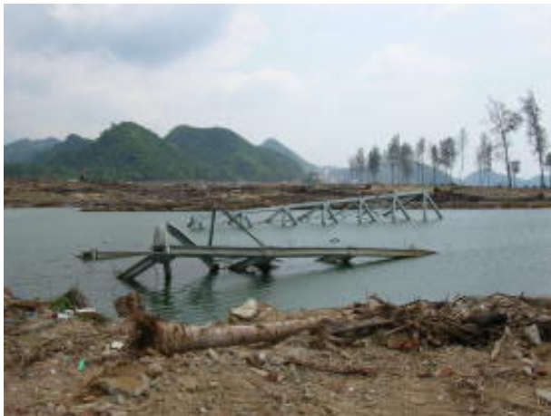
Photo 11.19 Washing out of Steel Truss
