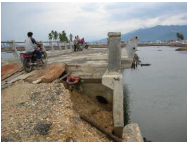
Photo 11.9 Lateral Displacement of Deck
