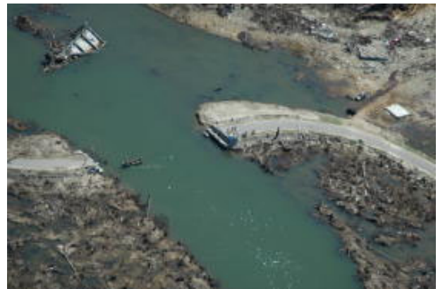
Photo 11.27 Washout of Truss Bridge (4) (courtesy of Aceh Provincial Government)
