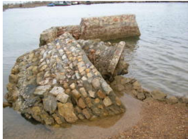
Photo 11.4 Masonry Substructure and Washout Effect of Surrounding Soils
