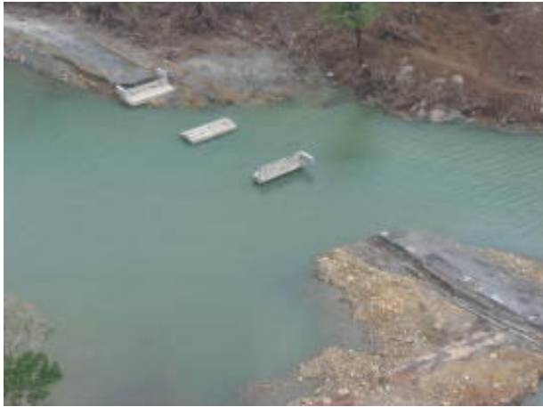
Photo 11.29 Washout of Bridge and Soil (courtesy of Aceh Provincial Government)
