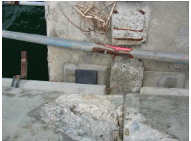
Photo 11.8 Rubber Sheet Type Bearing and Lateral Displacement at Bearing
