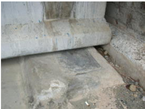
Photo 11.7 Lateral Displacement of Deck
