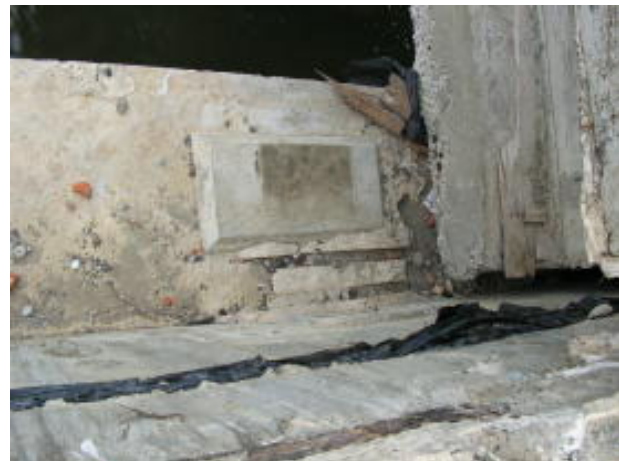
Photo 11.10 Displacement at Bearing
