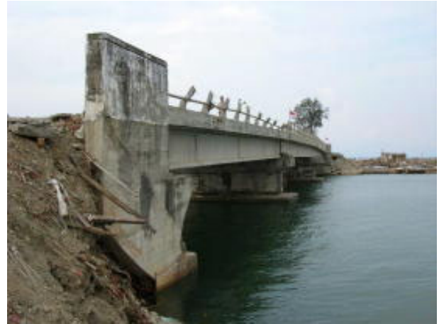
Photo 11.6 Washout Effect of Backfill Soils
