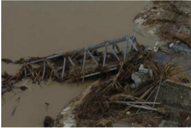
Photo 11.24 Washout of Truss Bridge (1) (courtesy of Aceh Provincial Government)
