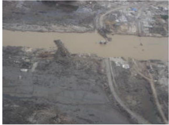
Photo 11.25 Washout of Truss Bridge (2) (courtesy of Aceh Provincial Government)
