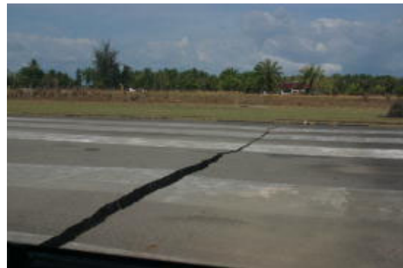
Photo 11.34 Damage of Airstrip (courtesy of Dr. Osumi)
