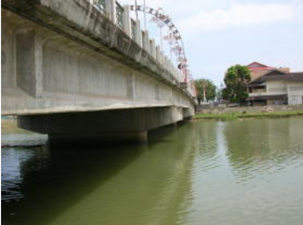
Photo 11.13 Bridge affected by Shaking
