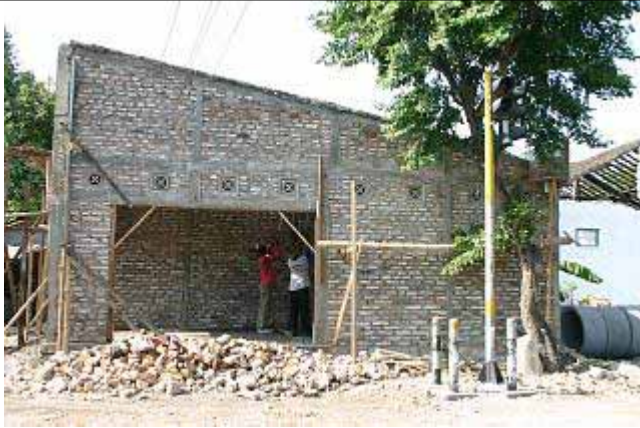
A shop (?) at a corner of crossing of a road leading from Bantul to Imogiri. RC frames confine brick walls.
