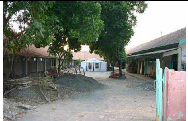
2006.09.16 New school on the left is under construction. The school on the right shows its original structure, No repair work has done yet.
