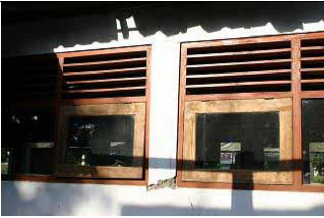
2006.06.12 cracks are found in the middle column
