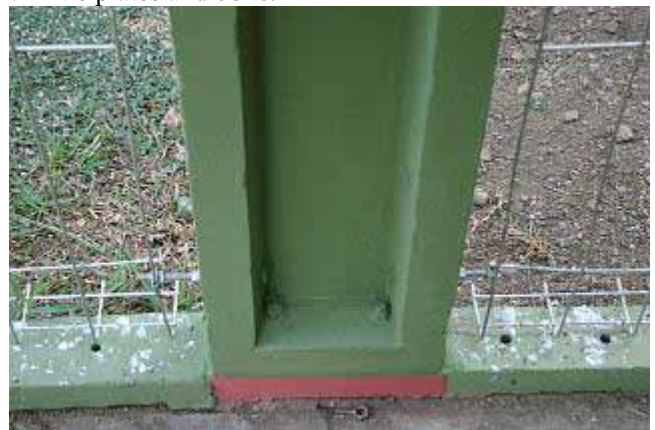
(d) A column is fastened upright with bolts at its bottom end to the foundation.
