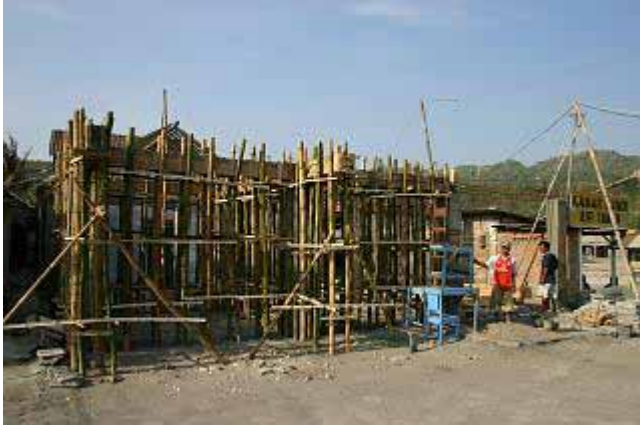
House at Parangtritis Beach. RC frame is observed.
