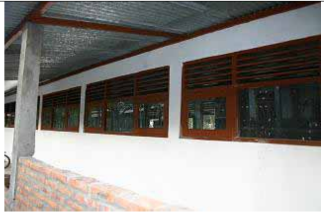
2006.09.16 Repaired, but method is unknown
