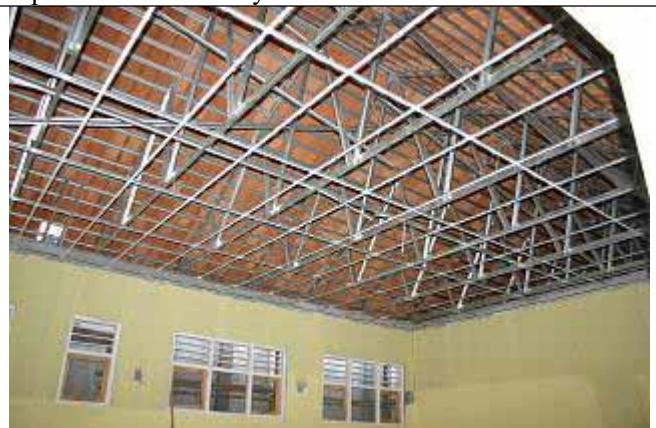
Roofing framework and beams along the top ends of walls are seen.
