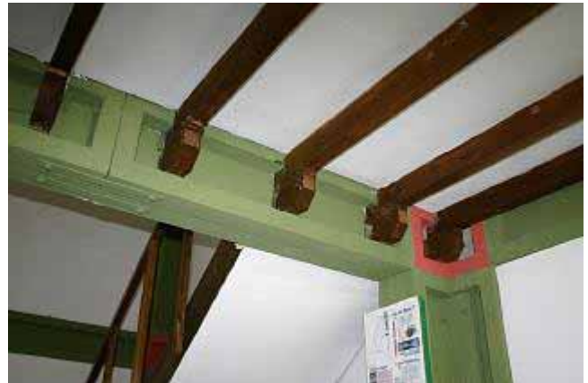
(b) Beam connection; Beams are fastened together with thin tie plates and bolts.
