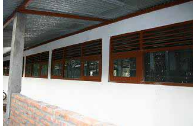
2006.09.16 Repaired, but method is unknown
