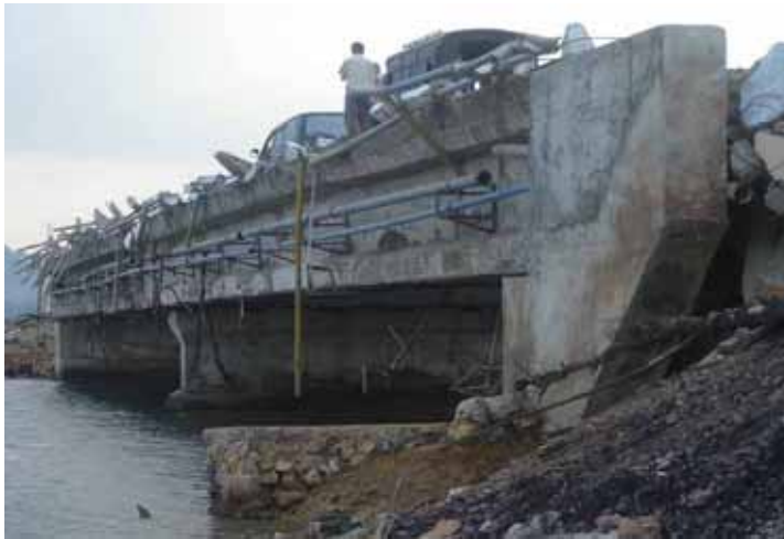
Figure 7. Asoe Nanggroe Bridge after the 2004 Tsunami
