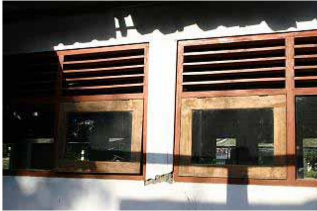
2006.06.12 cracks are found in the middle column
