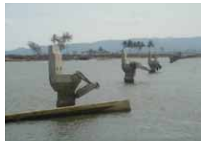
(c) Washed Away Girders
