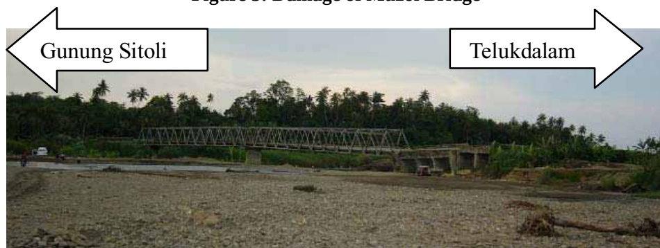
Figure 6. Damage of Idano Gawo Bridge
