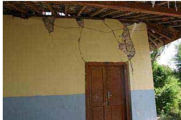
Damage to corner wall
