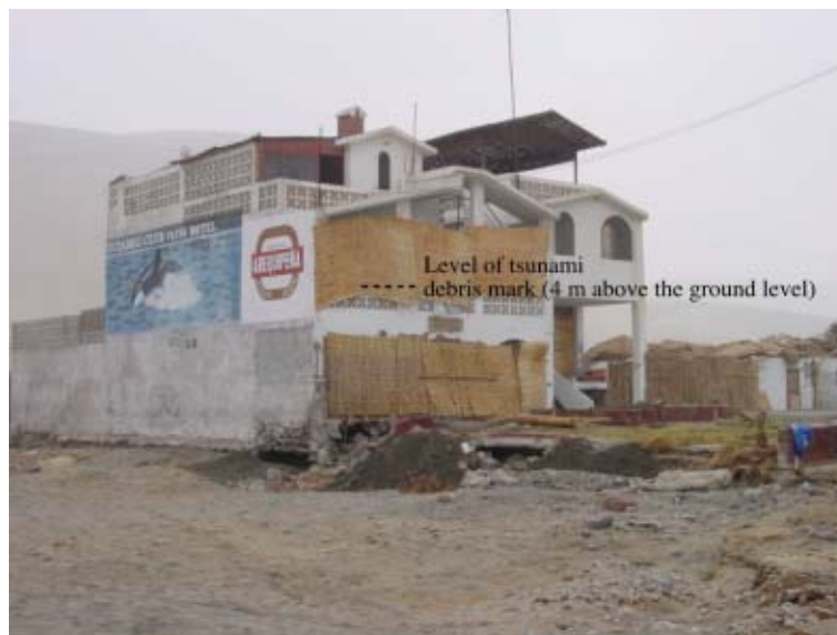
Figure 6.6 Hotel building struck by the tsunami at La Punta
