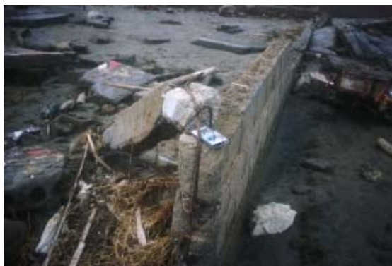
Figure 6.19 Reinforcing bars bent by tsunami.
