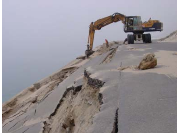
Figure 6.3 Damaged Pan American Highway near Ocona
