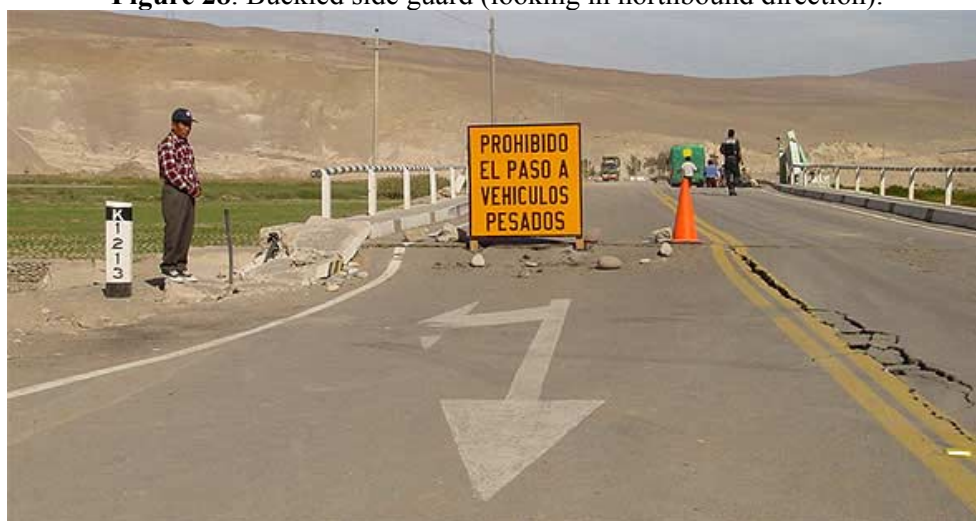
Figure 29. Settlement of bridge approach and cracking of road. Only one lane is open for traffic (looking in southbound direction).
