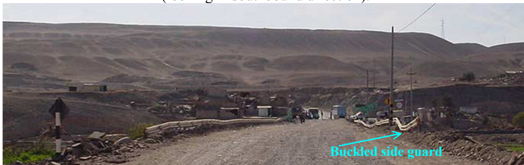
Figure 28. Buckled side guard (looking in northbound direction).
