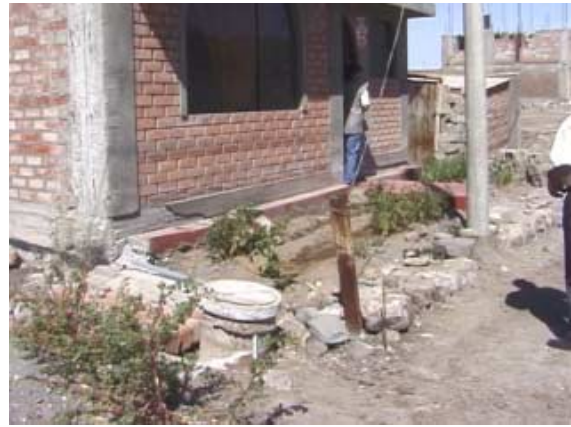
(d) Uplift of sewage catch basin located near drainage channel
