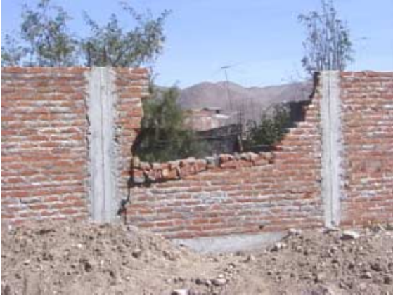
(a) Collapsed brick wall due to lateral spreading
