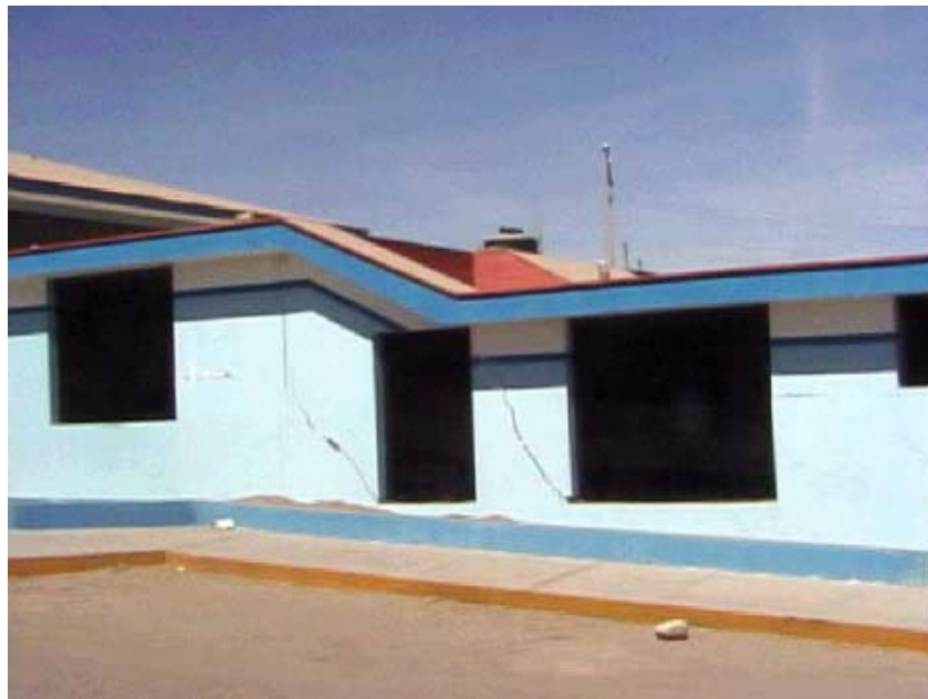
Figure 18. School constructed on expansive soil layers
