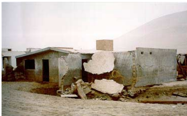
Figure 20. Destroyed dwellings by tsunami
