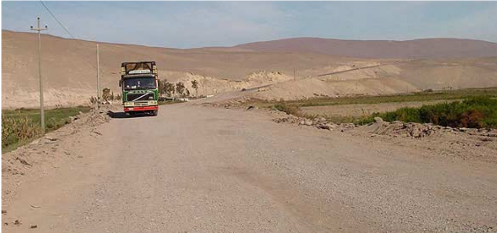
Figure 27. Pan American Highway Pavement removed after damaged due the earthquake (looking in southbound direction).
