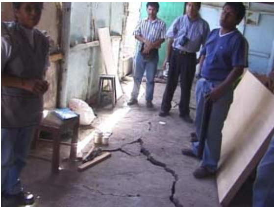
(e) Heave of house floor due to sand boil
