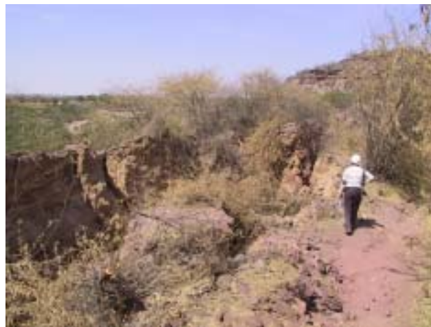
Figure 6.6 Settlement and slumping of Chang dam
