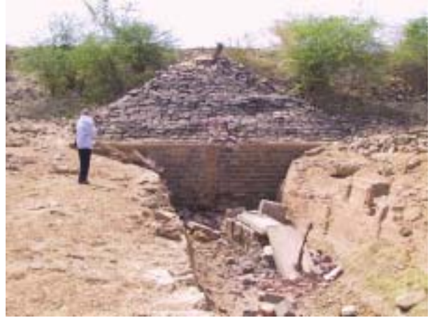
Figure 6.9 Failure of water intake tower
