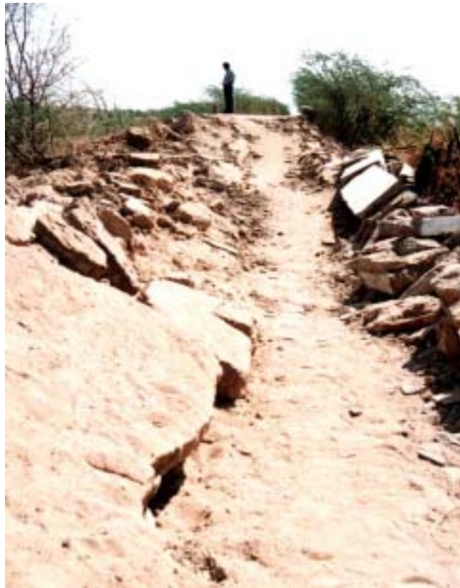
Figure 6.3 Settlement and slumping of Suvi dam towards upstream side
