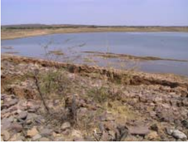
Figure 6.8 Upstream slope failure due to liquefaction
