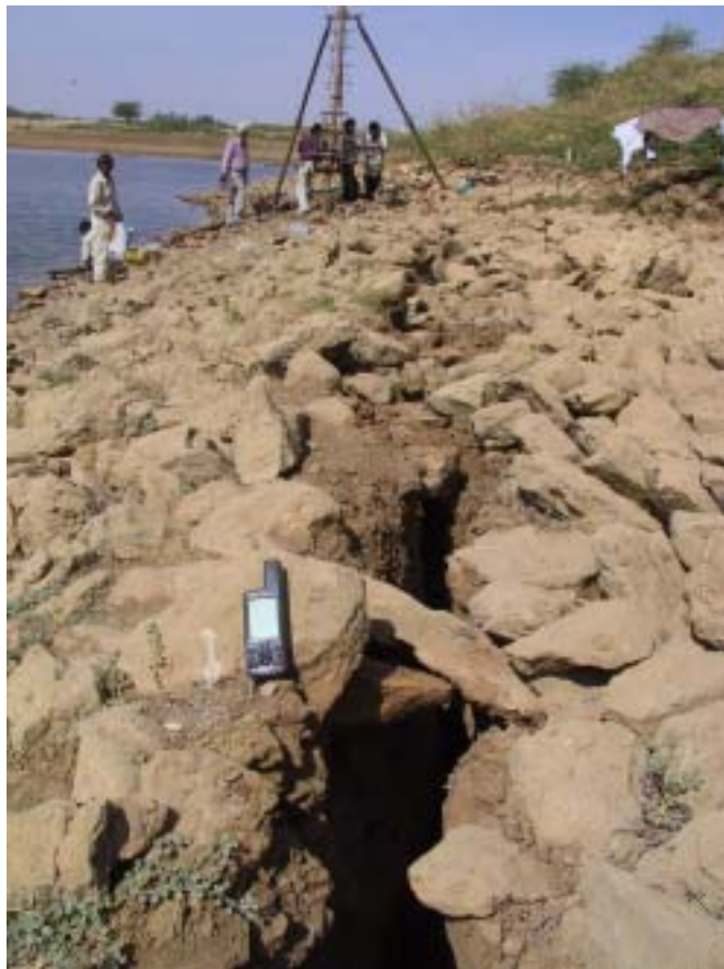
Figure 6.5 Large crack at the boulder toe.
