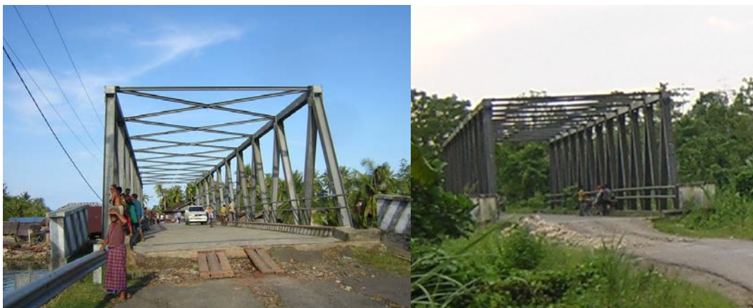
Figure 10.7 Settlement of approach embankments of bridges
