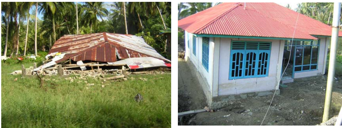
Figure 9.3 Collapsed of heavily damaged single RC story buildings
