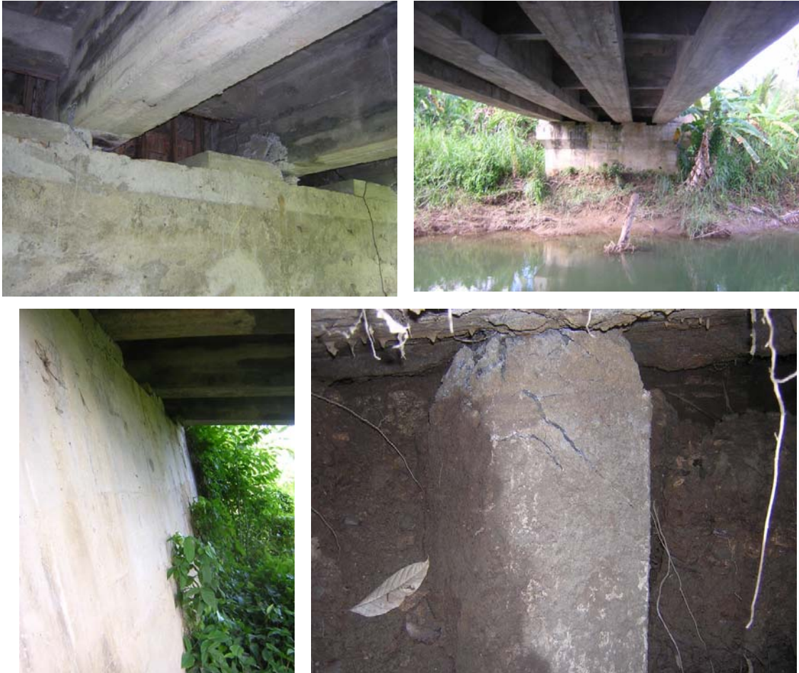
Figure 10.5 Some examples of damage to RC bridges
