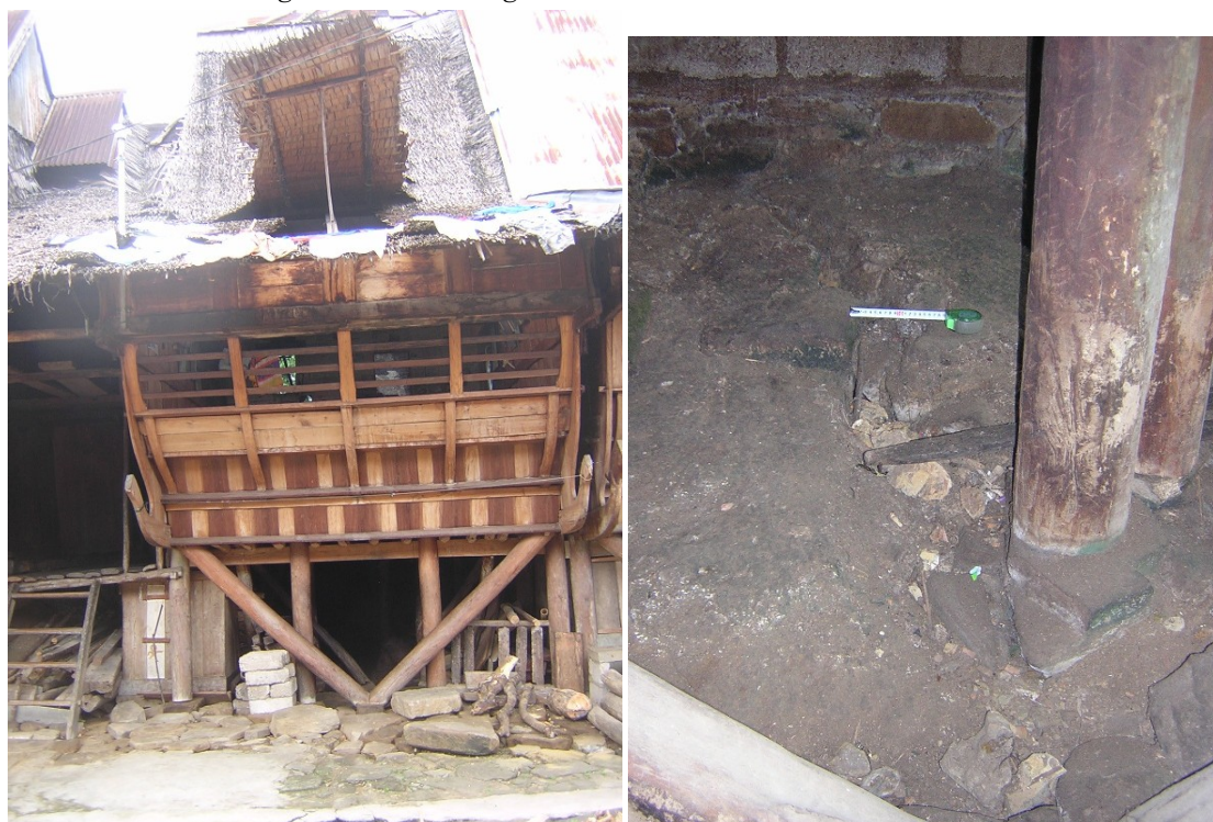
Figure 9.12 A traditional Nias house and a crack in ground at its basement
