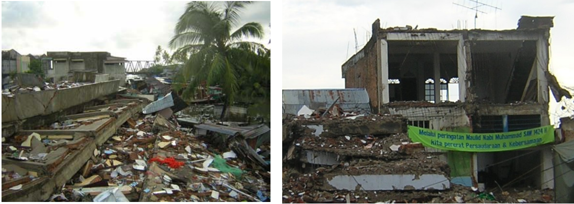
Figure 9.4 Out-of-plane failure of infill walls
