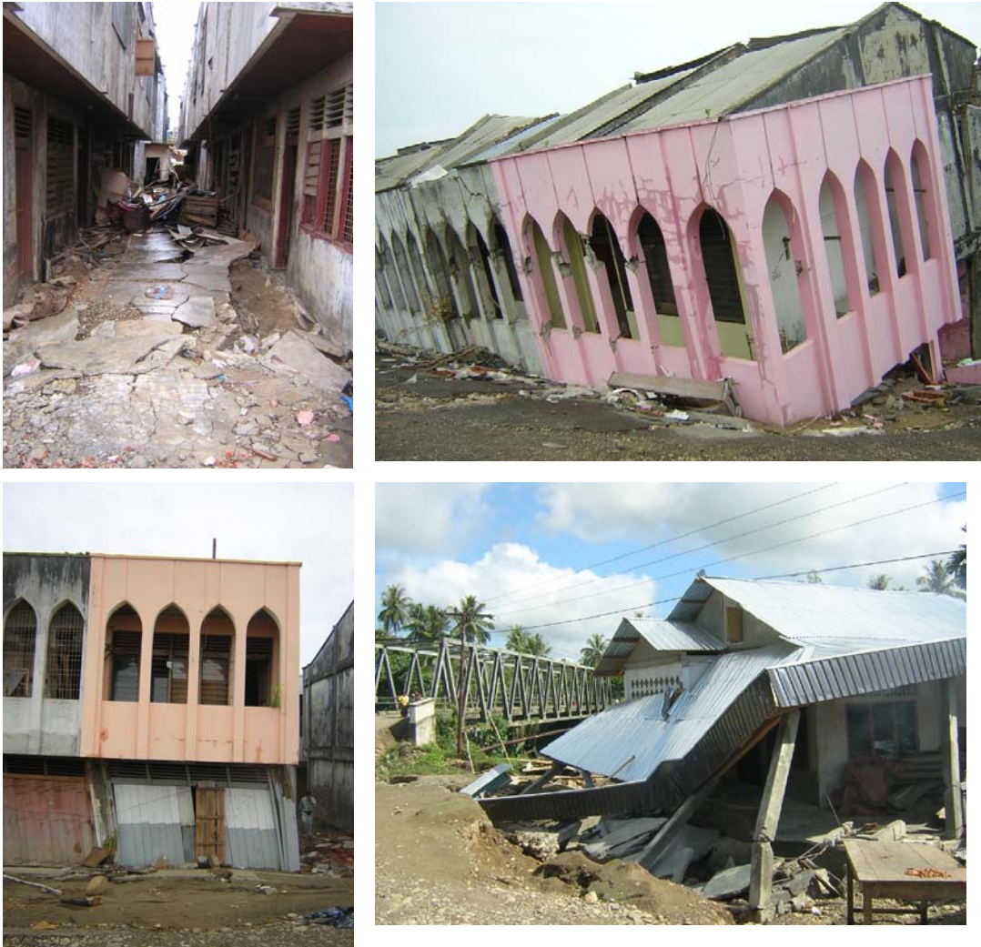
Figure 9.1 Liquefaction induced damage to buildings in Adapazari
