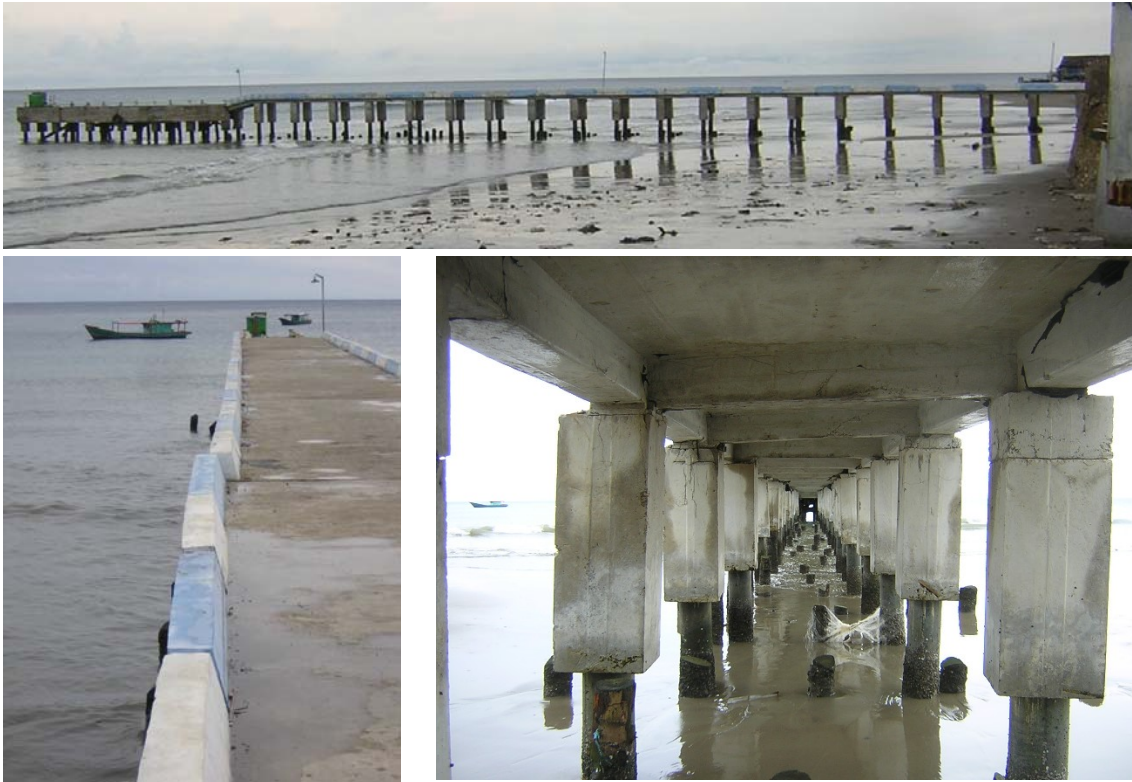
(a) Damage at Gunung Sutoli port
