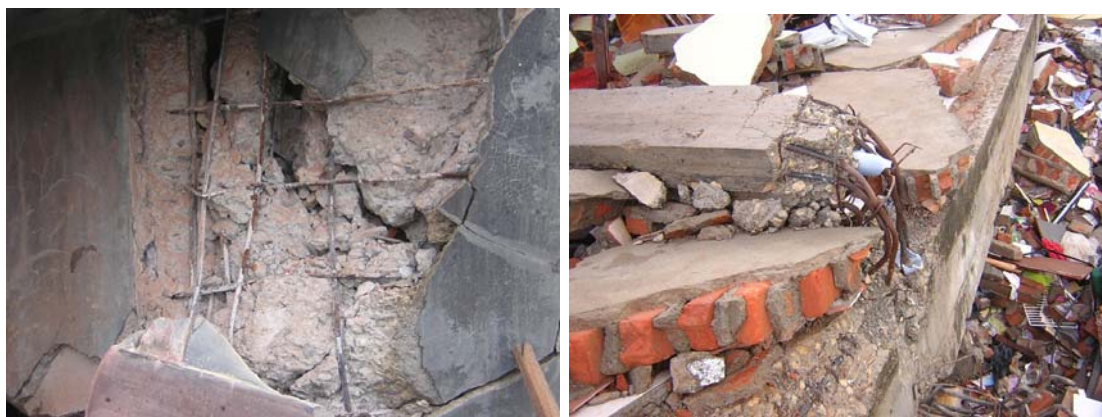
Figure 9.9 Corrosion of steel bars and non-cleaned sand and gravel
