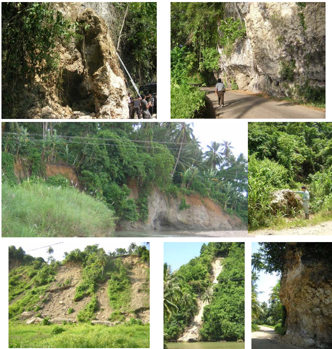
Figure 12.1 Various slope failures along inspected routes
