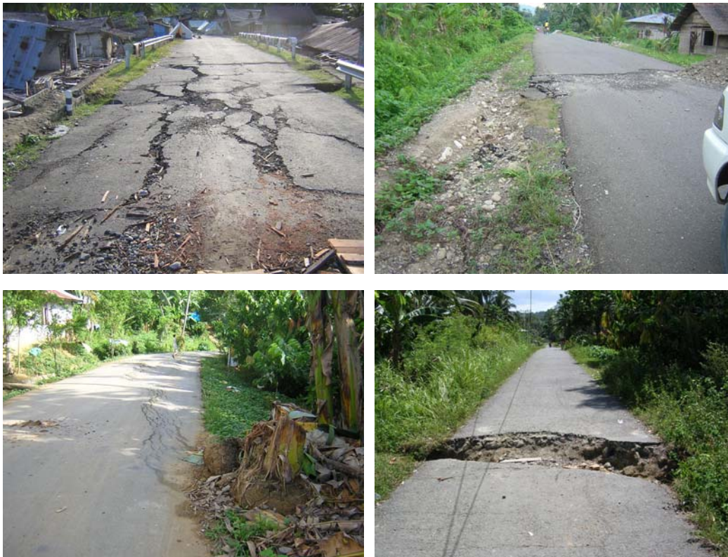
Figure 10.1 Damage to roads
