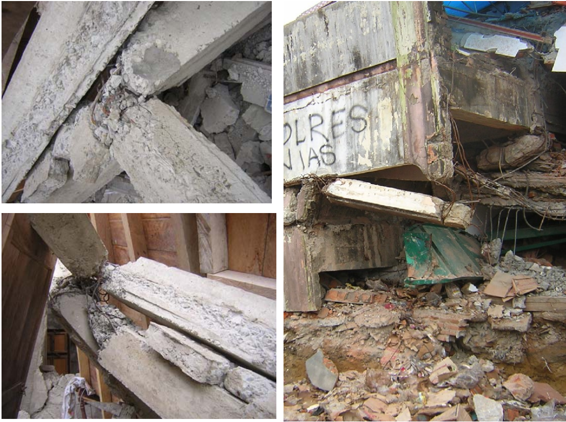
Figure 9.6 Typical poorly constructed column-beam joints
