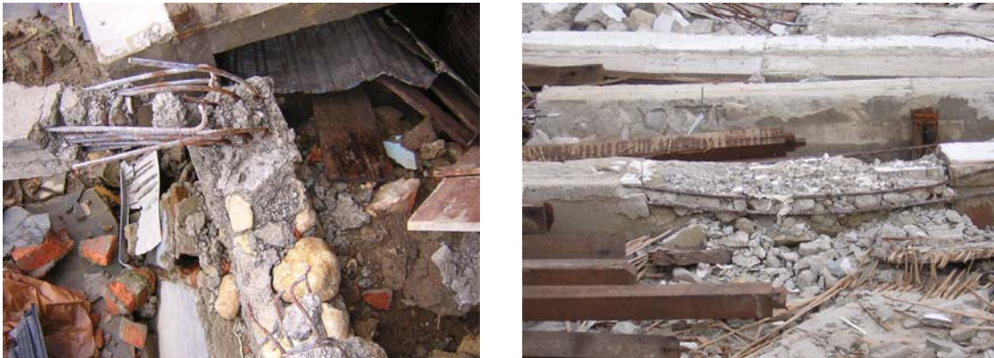
Figure 9.5 Thin stirrups with too large spacing and large boulders in a column
