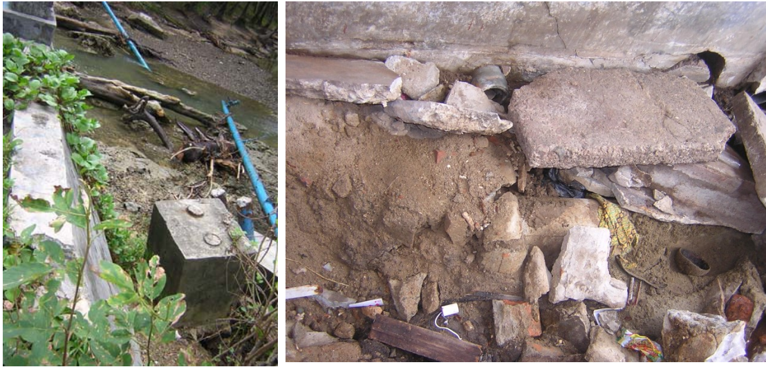
Figure 14.2 Views of damage to water pipes and sewage
