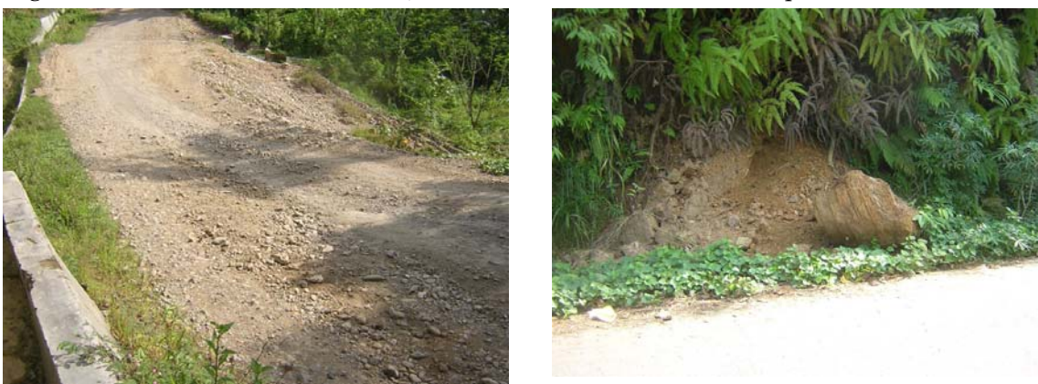
Figure 12.3 Some slope movements and rockfall in weathered soft sedimentary rocks
