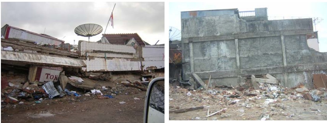
Figure9.7 Failure of buildings due to soft floor effect
