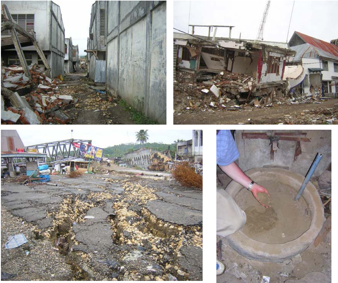
Figure 9.2 Effects of liquefaction and lateral spreading on RC buildings
