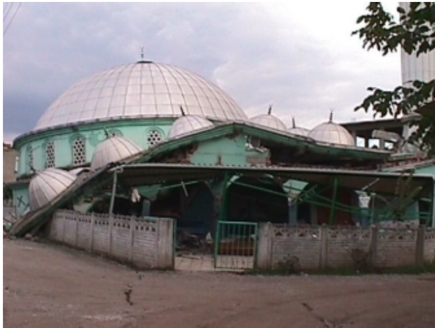
Figure 10.1 Totally collapsed mosque at Kavaklı district of Gölcük
