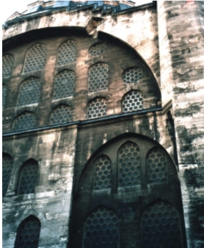
Figure 10.5 A view of damaged Mihrimah Sultan Mosque
