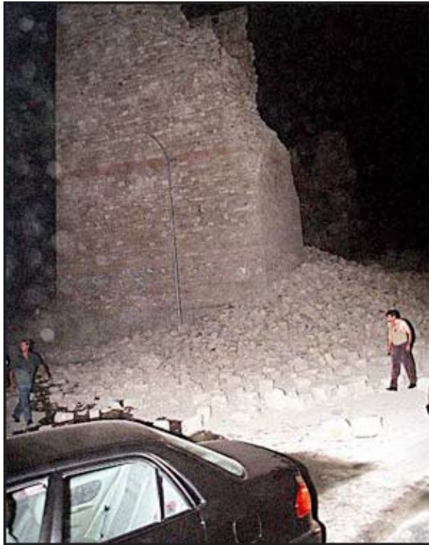
Figure 10.6 Partial collapse of Istanbul City Wall (Surlar)
