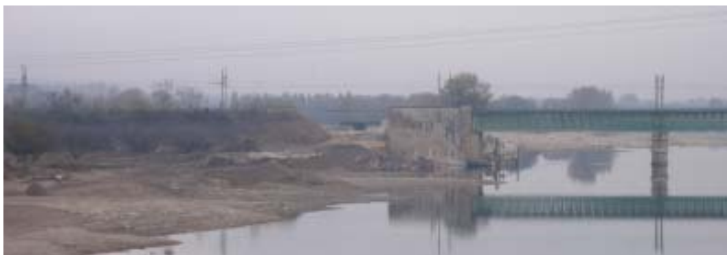
Photo-4 Damages on railroad bridge (fillings around the abutment have been washed away)
