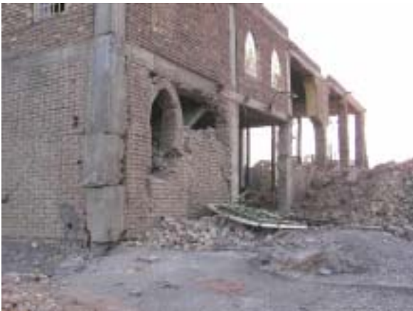
Photo-3: A damaged mosque
