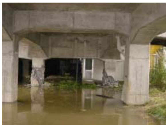
図-18 損傷状況 (R2-1)
