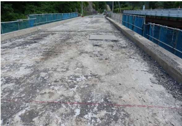
Photo B Pulverized concrete on reinforced concrete deck
