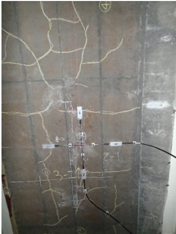
Photo A Grid-like cracking on underside of deck
