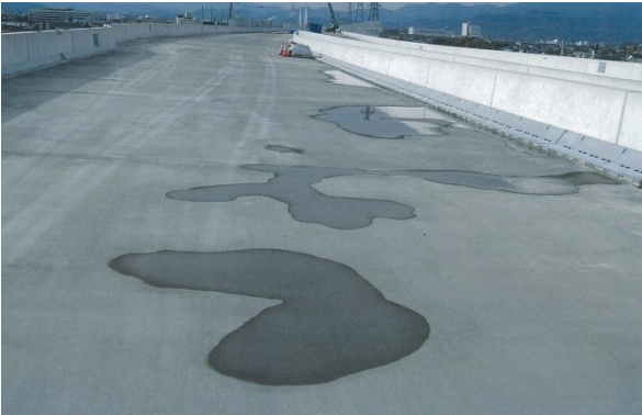
Photo E Water collects on deck after rain
