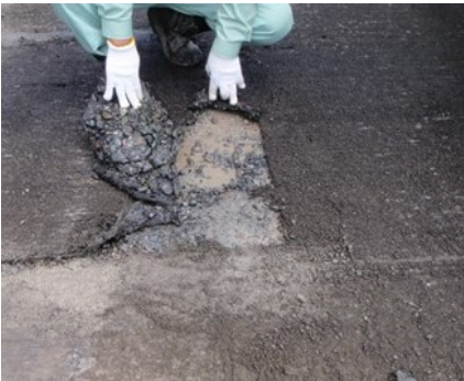
Photo D Water collects under waterproofing layer
