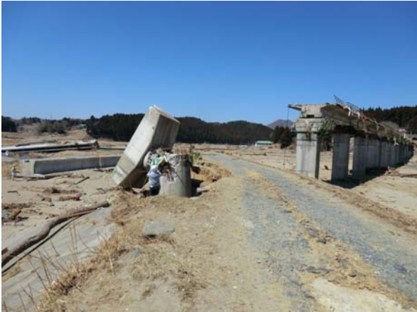
Fig.4 Failed pier (Tutanigawa bridge)
