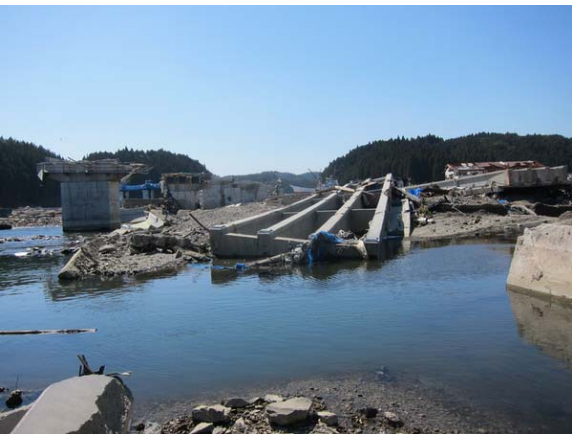
Fig.9 Falling down of PC girders (Utatsu-ohashi bridge)
