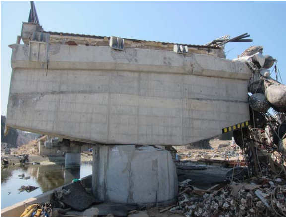
Fig.10 Rupture of devices
