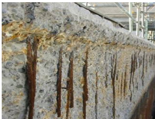
Photograph-1 Corrosion state of reinforcement after removal of deteriorated portions
