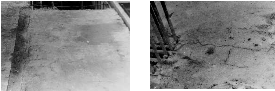
Figure 5 Surface cracks of concrete structures due to plastic deformation
