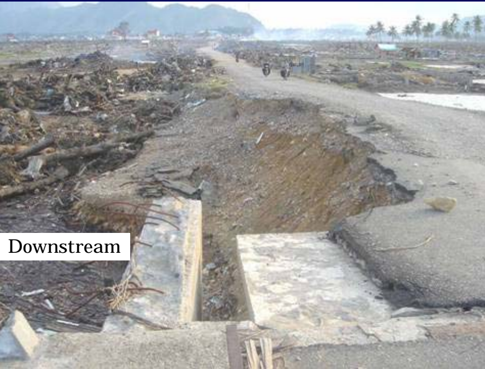
(Scouring at Southern Approach)
