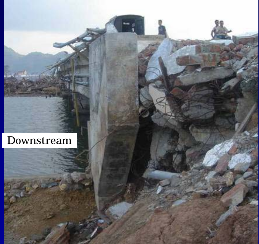
(Scouring at Northern Approach)
